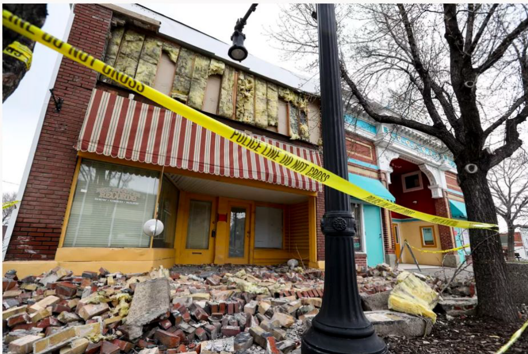
Caution tape surrounds a damaged building on Magna's Main Street on Tuesday, March 24, 2020, following a 5.7 magnitude earthquake that was centered near the city on March 18. The street is now open to traffic. | Steve Griffin, Deseret News Utah just experienced a 5.7 earthquake. Here's what a 7.0 would look like (Article)
